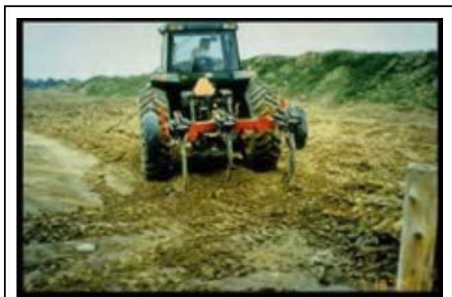
Fig. 9. This medium tractor is pulling a 3-shank deep ripper. The severely compacted construction access corridor is narrow, and the 120 hp tractor is more maneuverable for Phase 1 deep ripping (subsoil fracturing), here.
