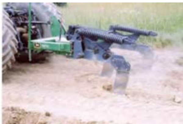
Fig. 10. An early pass with a 3-shank deep ripper penetrating only 8 inches into this worksite's severely compressed subsoil.
